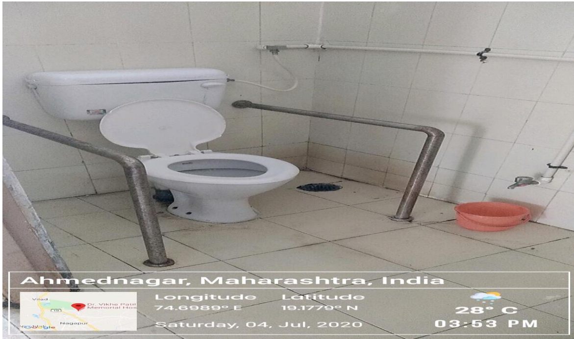
Washroom facilities for Disabled Person
